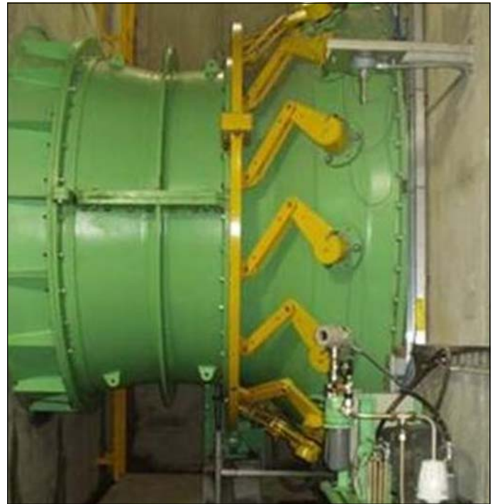
One of the project's 7.5 MW horizontal Kaplan turbines
