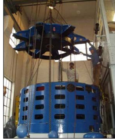
GMP realizes increased energy benefits from unit overhaul
