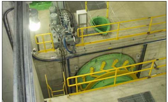
Interior of powerhouse looking down on unit
