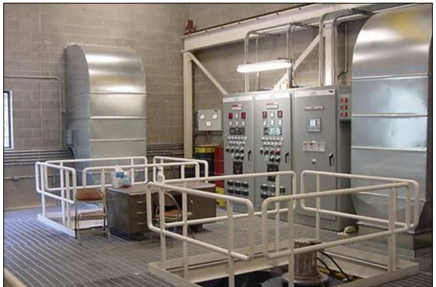
New powerhouse interior showing controls
