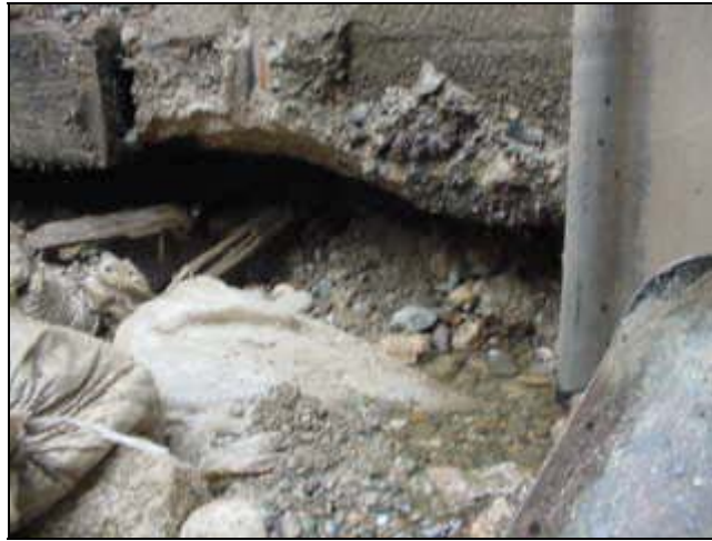
Void under existing concrete training wall discovered during dewatering. Note embedded sand bags.
